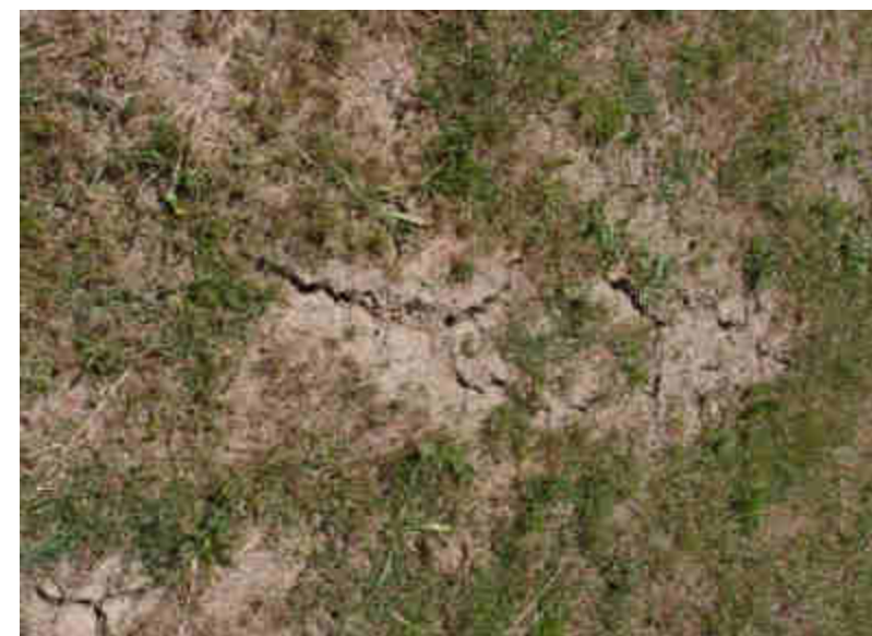
A picture of the silty soil with cracks and grass.
