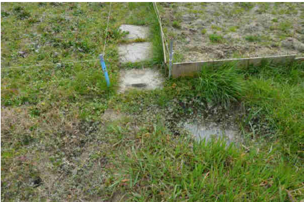
Figure 15: A depressed area in the neighbor lot shows some water accumulation.
