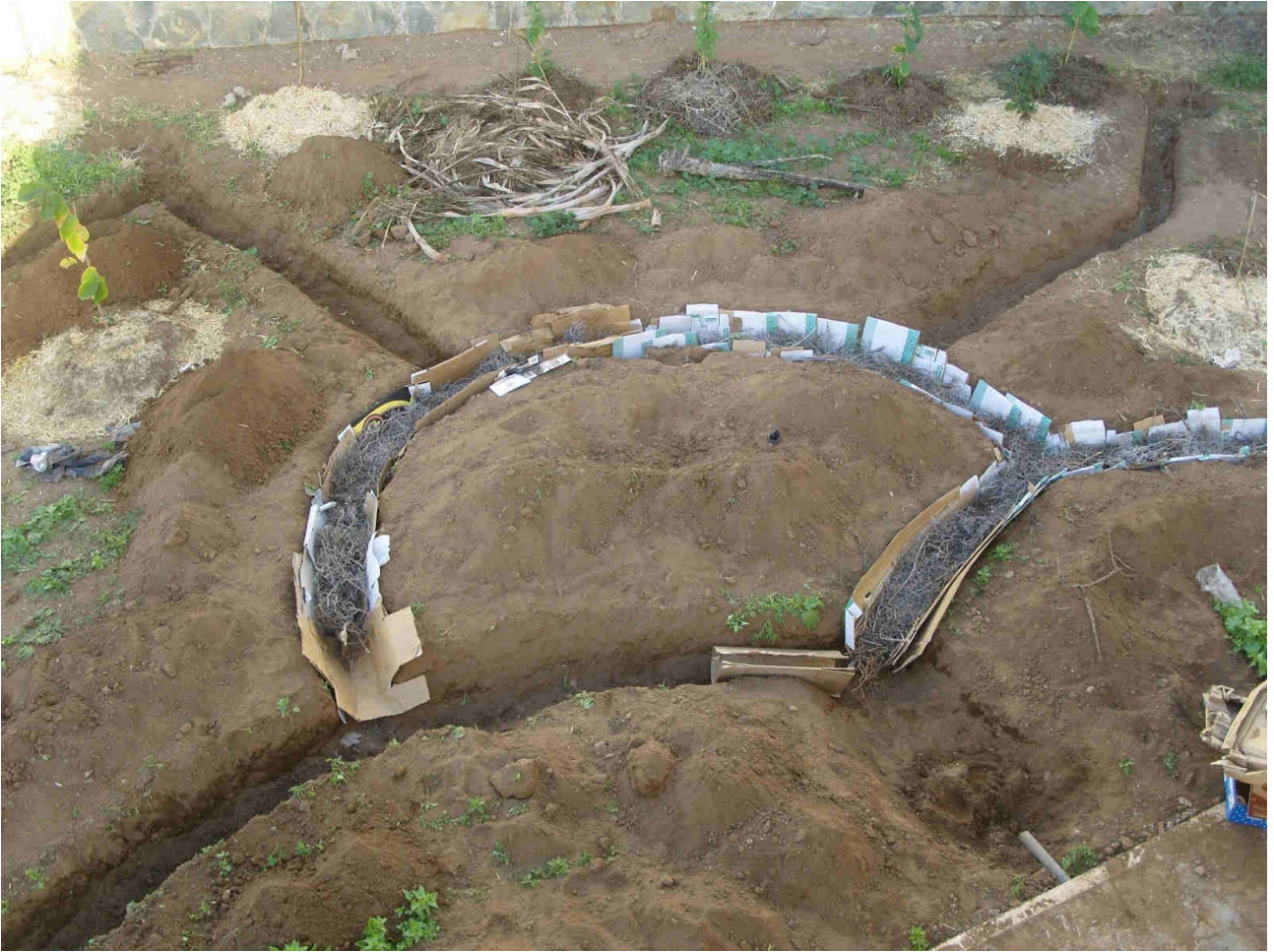
Figure 8: Bio-roll system. This system brings water and humidity in the garden area.
